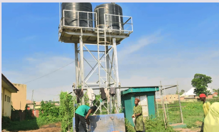
A solar-powered borehole facility installed at the renovated Gombe Abattoir by the Gombe L-PRES Project.
